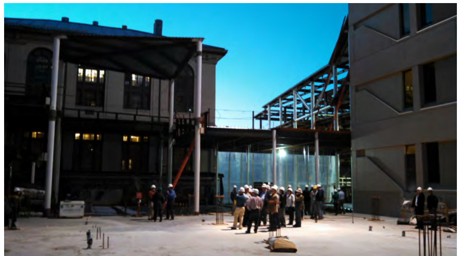
Scott Hall will actually squeeze between Wean Hall (right) and Hammerschlag Hall (left)
